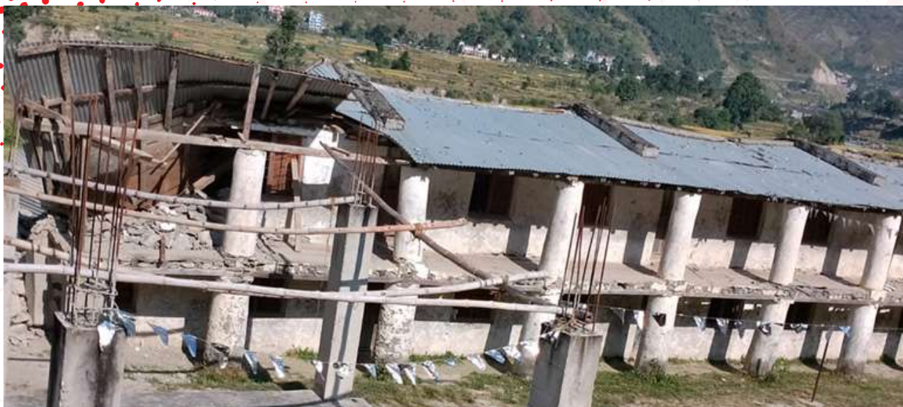
Figure 6. Bal Bikas Secondary School Building damaged by earthquake
