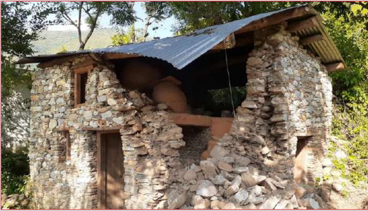
Figure 3. New house damaged by earthquake, Kuch Village.
